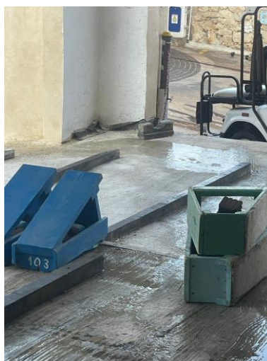
Figure 5: Area of overflow
