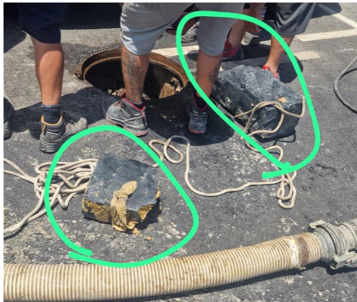
Figure 1: Material removed from the sewer line
