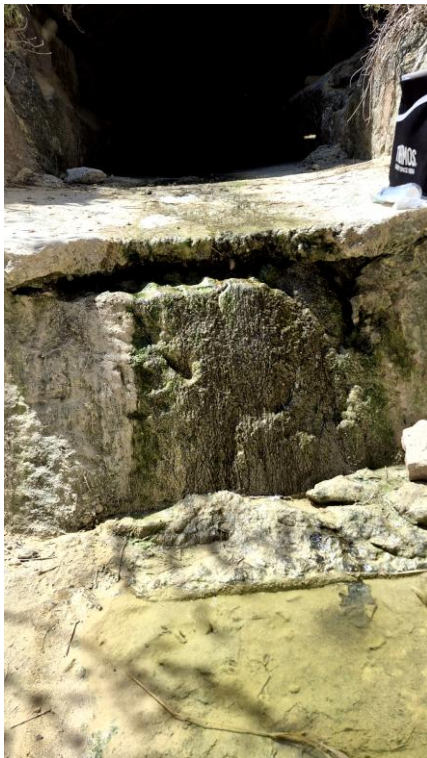
Figure 1: foul water form tunnel
