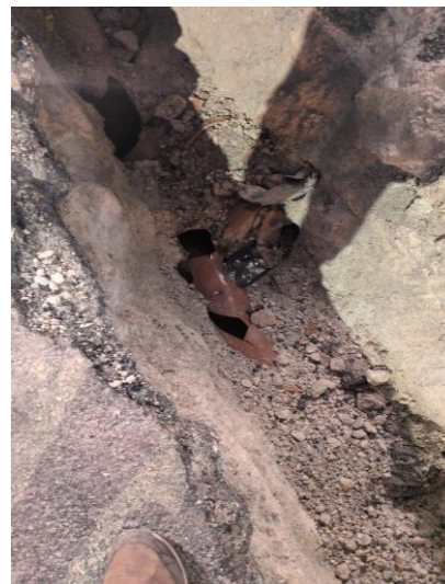
Figure 5: damage in main sewer
