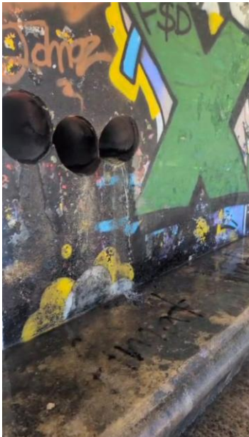
Figure 1: Origin of overflow into the sea
