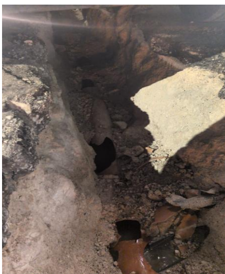
Figure 4: damage in main sewer
